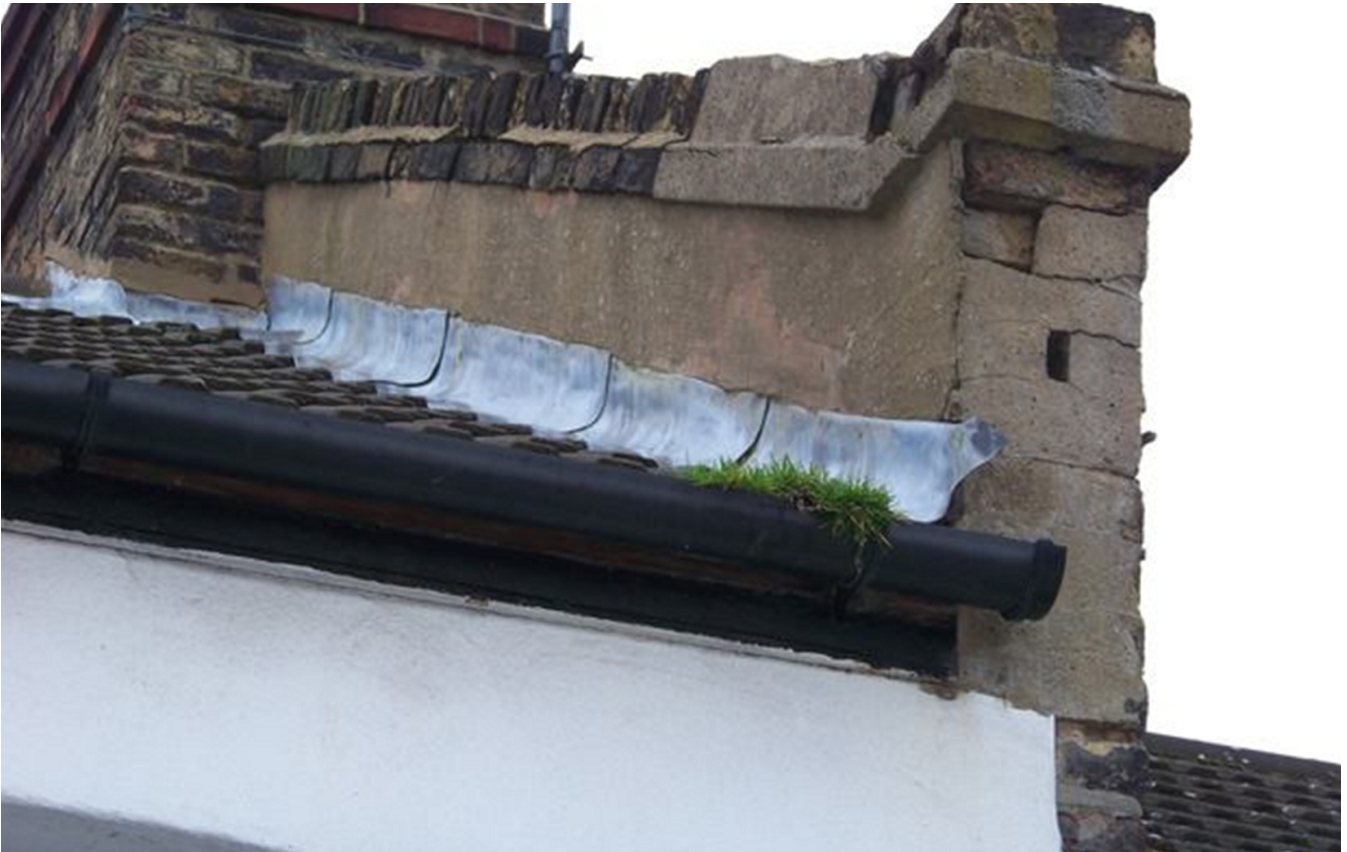
Figure 1: Parapet wall in poor condition (image © PCA)
