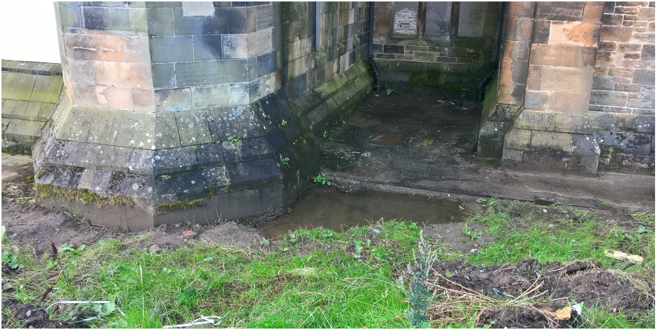
Figure 3: Defective rainwater disposal (image © Historic Environment Scotland)
