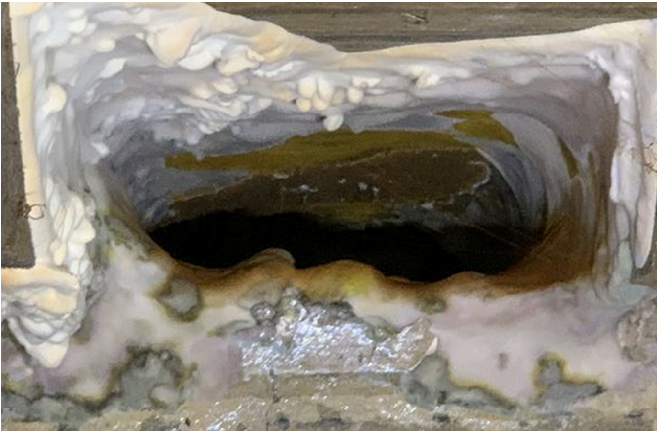
Figure 6: Dry rot under a suspended timber floor (image © RICS)
