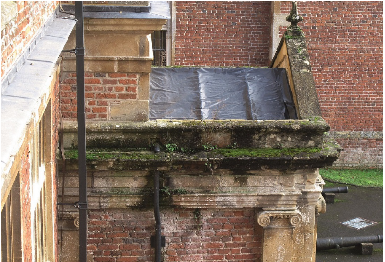
Figure 7: Poor maintenance (image © Historic England)
