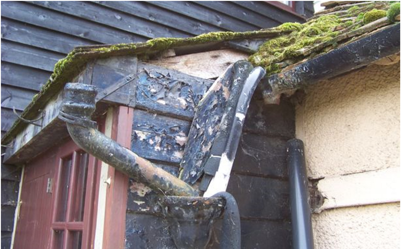
Figure 5: Defective rainwater gutters and downpipes (image © PCA)
