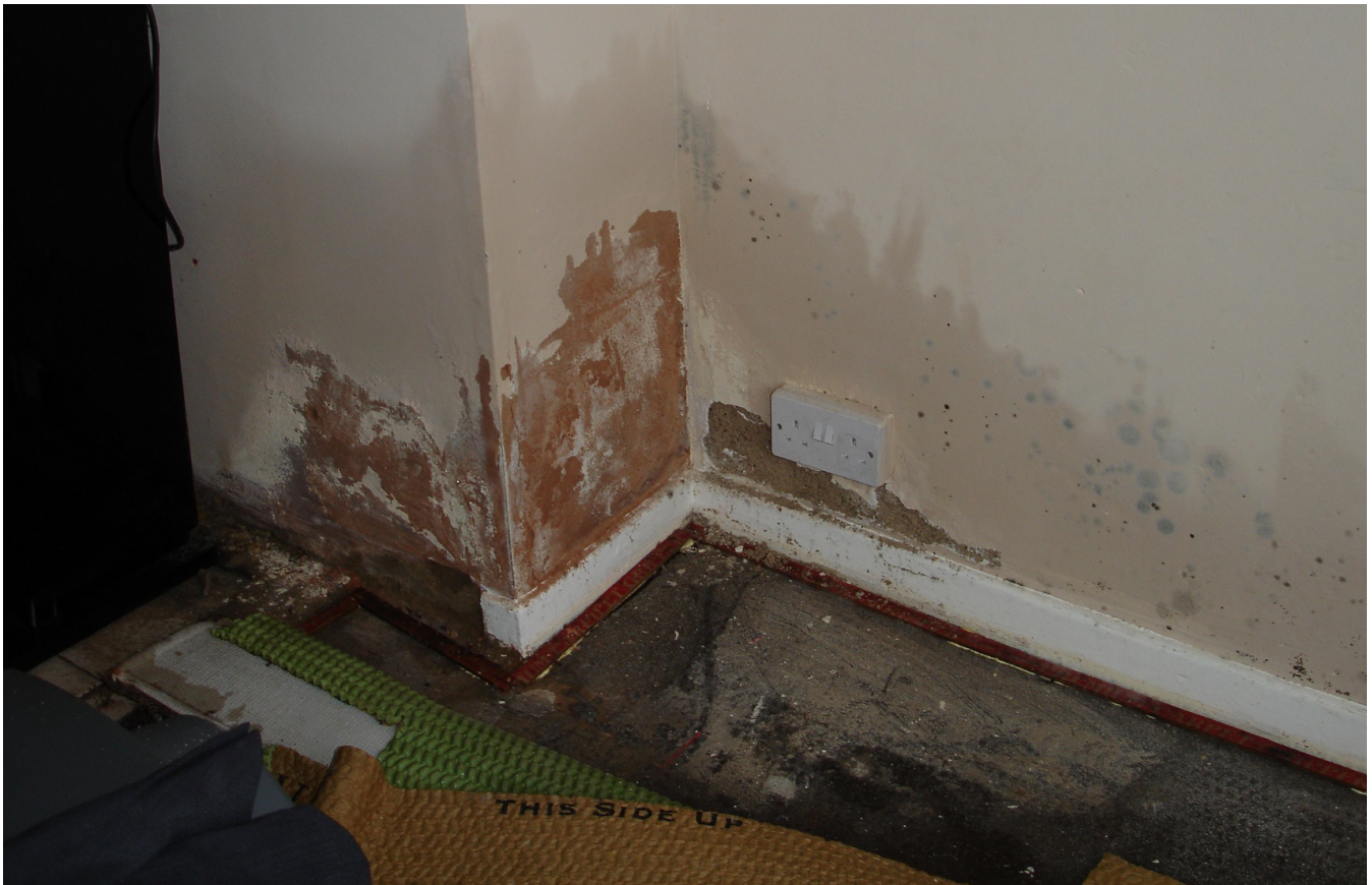
Figure 4: Elevated moisture in a wall (image © PCA)
