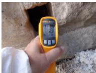
Surface temperature of steel frame above dew point with blown fibre CWI installed!
